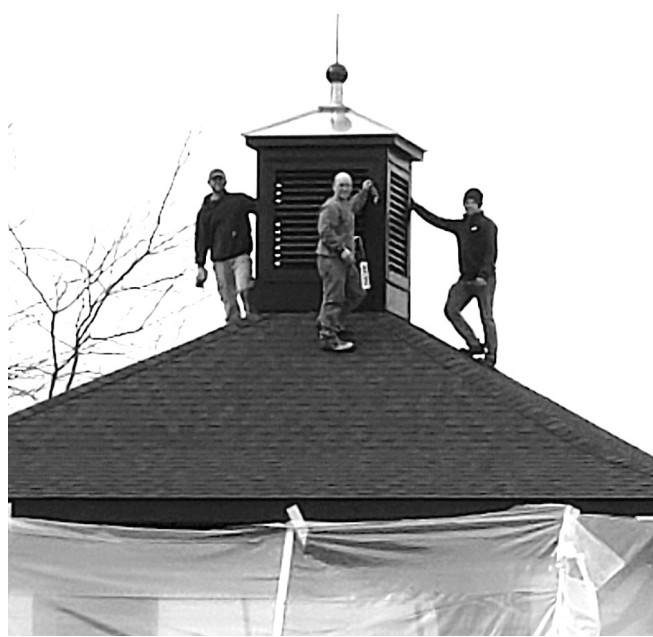
The Kroondyk Construction crew puts finishing touches on the pavilion cupulas on March 19. Courtesy photo
